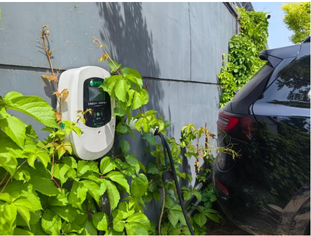
Factory electric vehicle charging station
